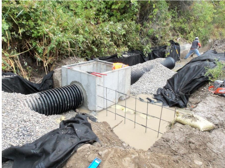
Placement of turn out box (rebar for cut off wall also shown)
