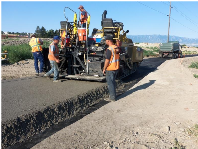
Placement of road base for the access road between 1200 E and the pressure reducing vault
