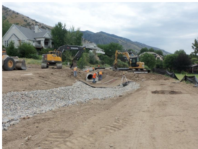
Construction of the culvert bridge connecting Lundstrom Park to the Bonneville Shoreline Trail
