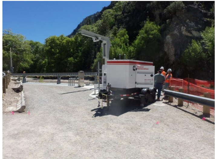
Portable generator at diversion
