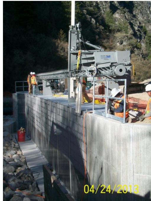
Installed Screen Cleaner
