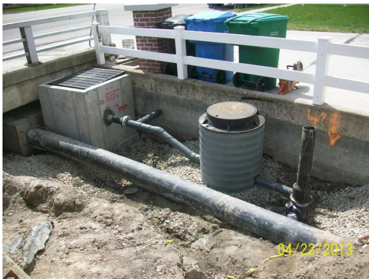
Turnout slightly north of the 400 N crossing
