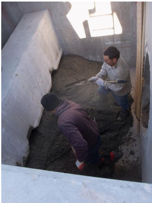
Pouring the sloped floor in the north bay of the pressure reducing structure
