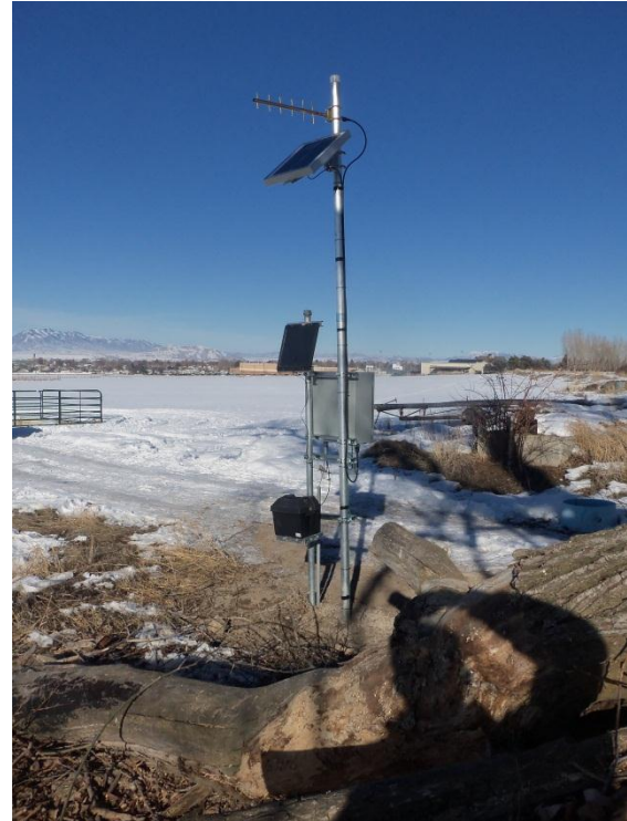
Metering equipment set up near 4700 N
