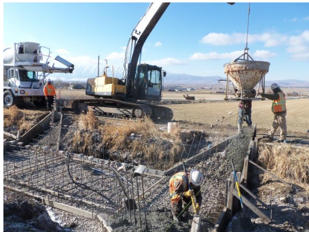
Placement of concrete for the floor slab on the lower 4400 N flume
