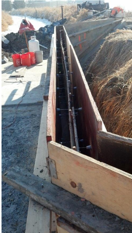
Wall forms and rebar ready for concrete on the lower 3100 N flume
