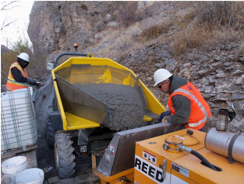
Delivering concrete to the small pumper to be transferred to the cast in place forms
