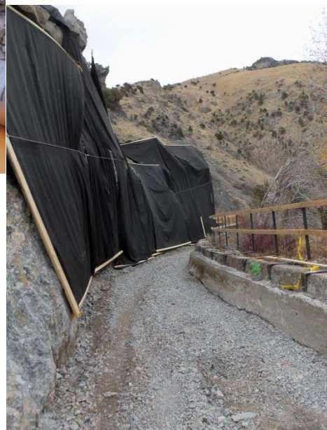
Rock Fall Protection
