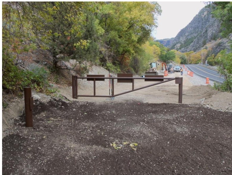
Pipe gate installed on east side of Canyon Segment
