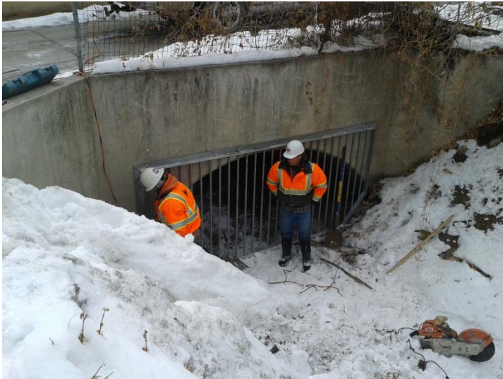
Placement of the grate over the dead end culvert near 400 N and 600 E
