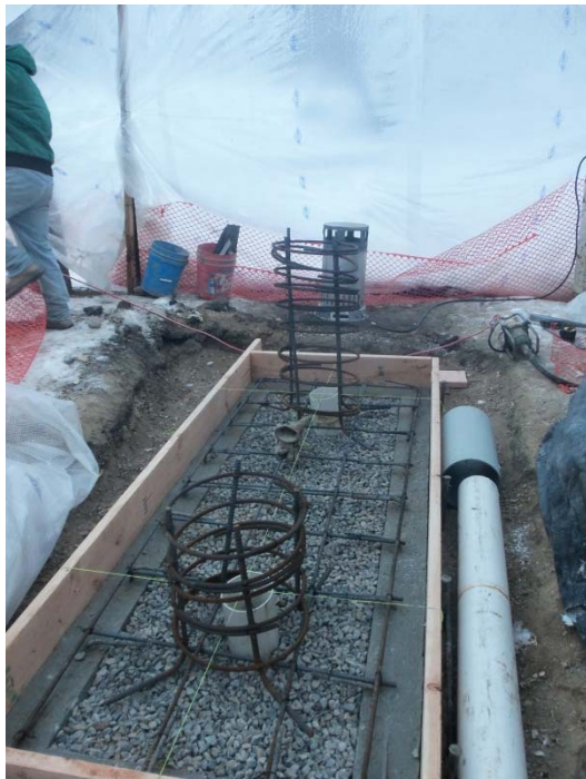
Placement of Rebar in the slab portion of the kiosk (spiral rebar for sign columns also shown)
